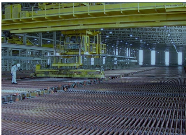
Electrolytic cells inspection and cathode extraction(Reference image).
